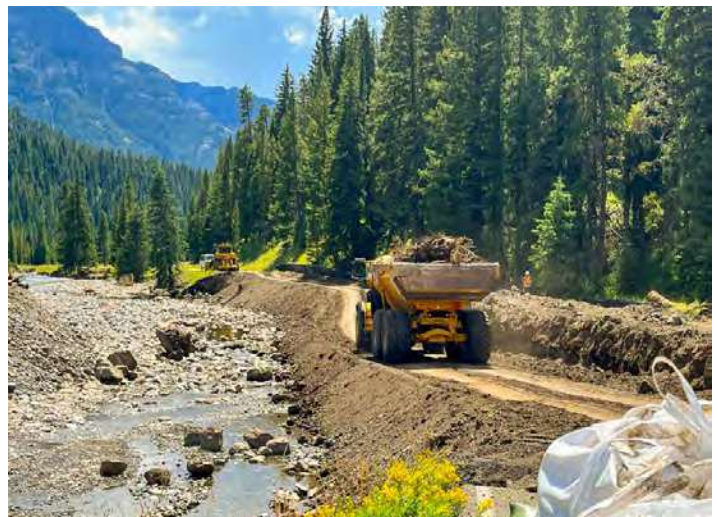
Below: A road crew works on the Northeast Entrance Road Improvement Project on August 15, 2022. Photo by Cam Sholly/NPS.
